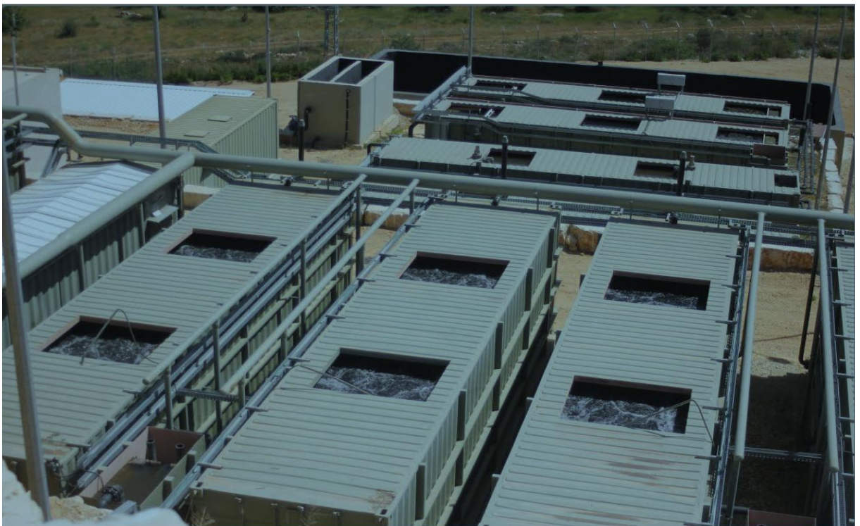
Figure 2.2: Rawabi wastewater treatment plant, containerized WWTP
